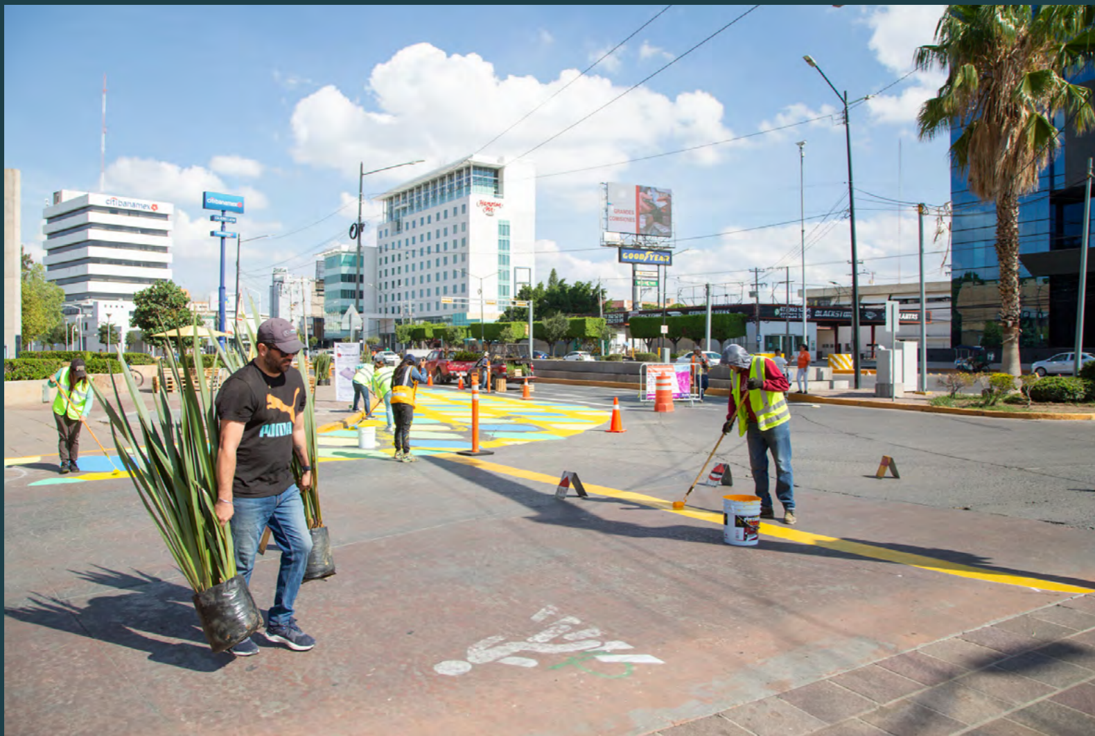
Improving pedestrian spaces between Blvd. Adolfo López Mateos, Blvd. Vasco de Quiroga and Calzada de los Héroes, July 2023. © WRI México
